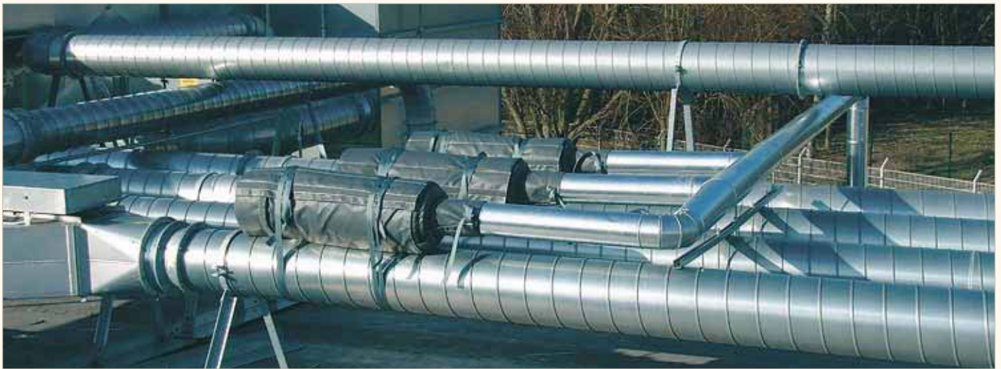
Anti-freeze protection of extinguishing devices with insulating bags
